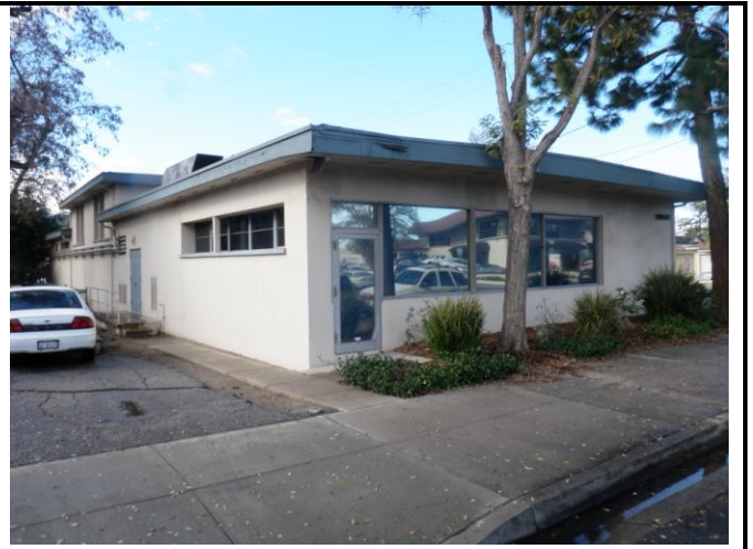
Photo 2: View of the northeast of the building; ACM window putty on the small windows
