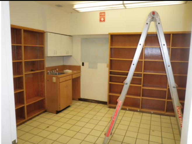
Photo 11: General view of the kitchen area, ACM tile is present under the white tile
