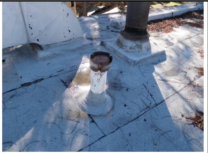
Photo 8: Asbestos cement vent pipe exhausting from the water heater
